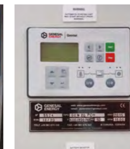
Panel de control
