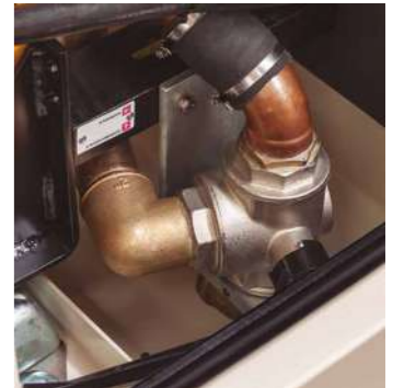
Selection valve for keel/radiator cooling
