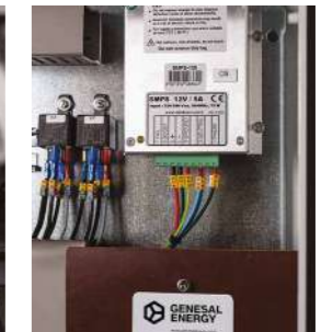
Engine battery maintainer from external grid
