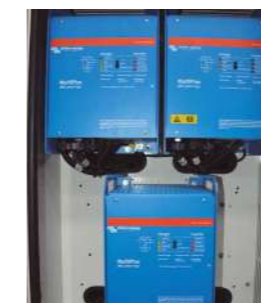
Battery inverters / chargers
