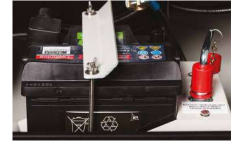
Battery with battery switch
